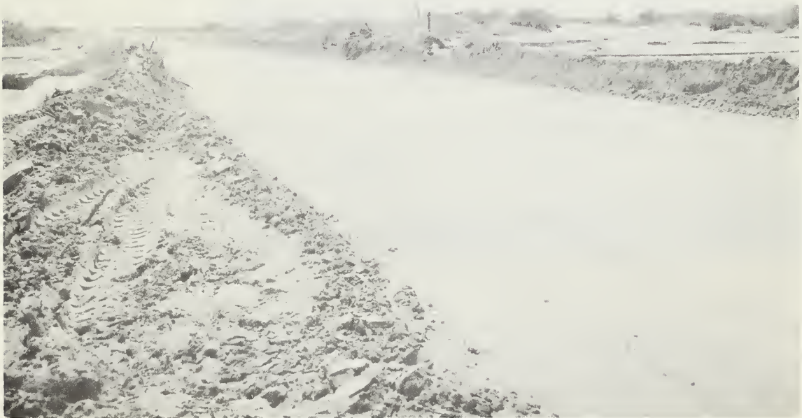
Highway 54 road damage Note sediment deposition.
